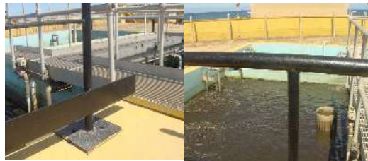
Figure 3. WWT Phase 1 complex of the GP1/ Z
